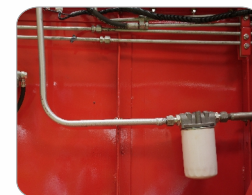
Double Oil Filters with Durable Steel Pipes
